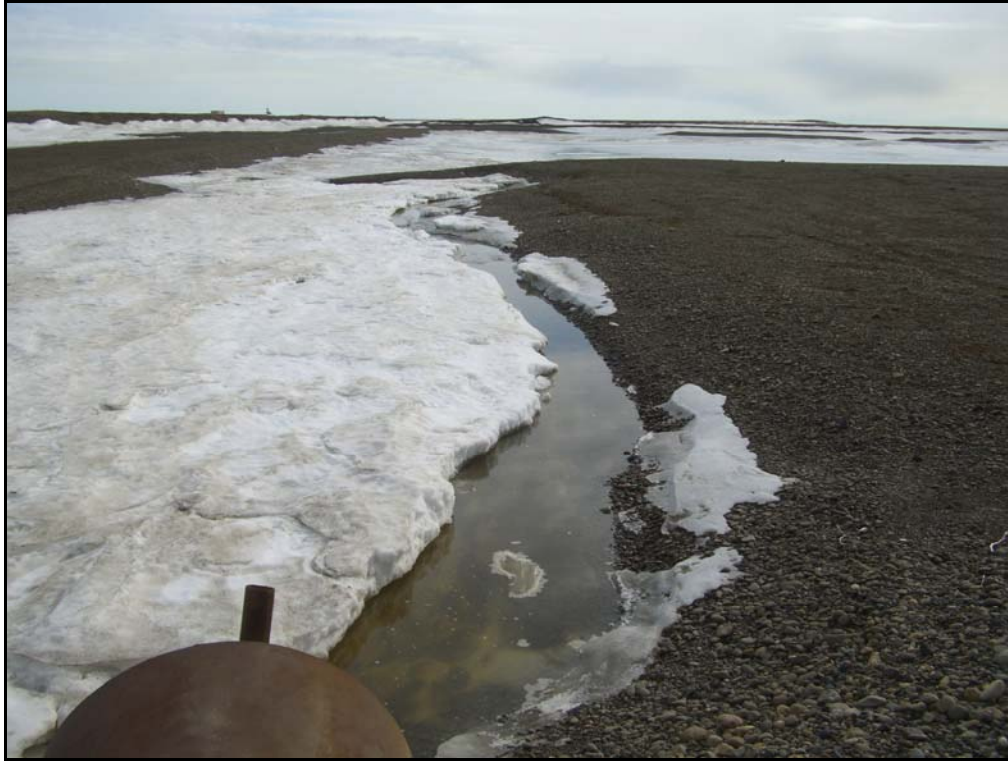
Figure 2. Culvert leading from Kuparuk Deadarm cell 1 into cell 2, photo by C. Cormack.
