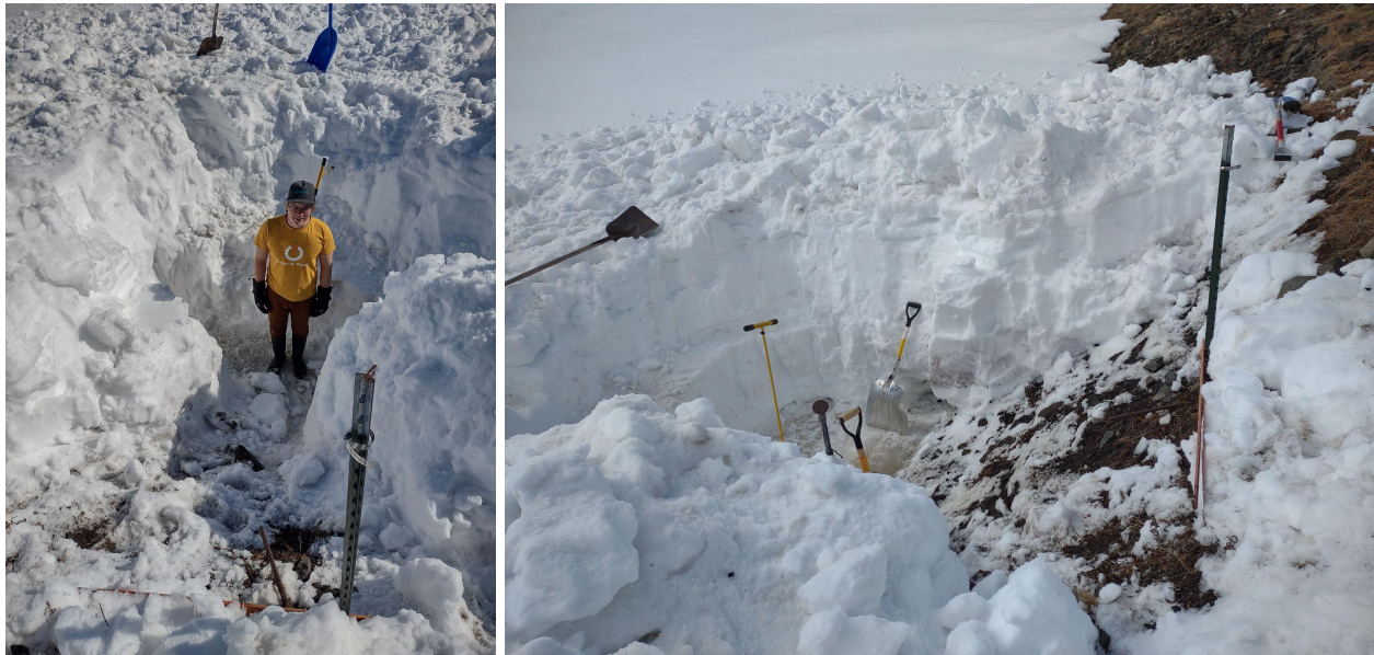
Left: The progress of clearing the culvert on the first day, with me for scale. Right: The progress on the second day. 5/18 & 5/19, Emily Youcha, UAF WERC
